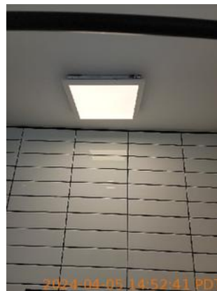
Exhaust Fan 📅 2024-04-05 14:52:41 🔍 45.4247589, -122.6263262 🖼️ Image
