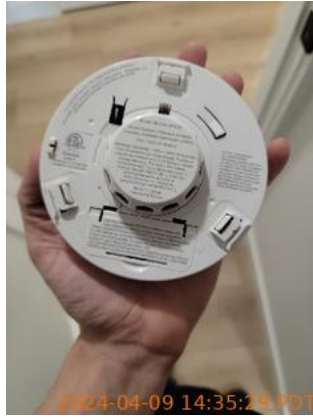
Smoke / CO detector
