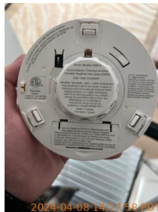
Smoke / CO detector
